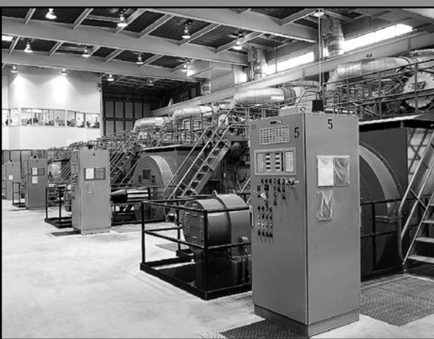
Central Generation facility at Plant No. 1, circa 1990s
