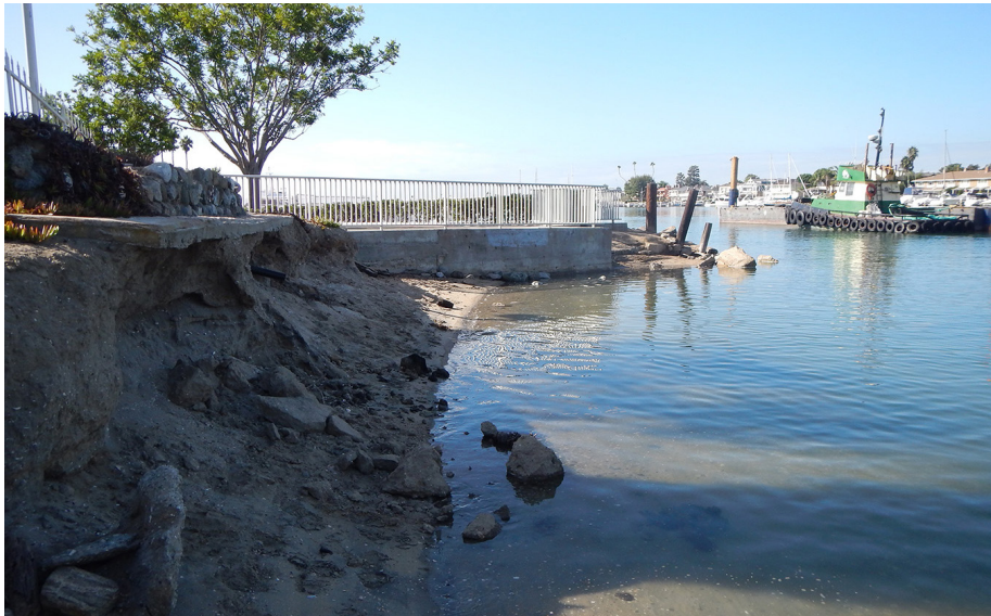
Photo 3. View looking south toward Newport Bay Channel, erosion along the eastern shore, and a seawall at the southern boundary of the project site.
