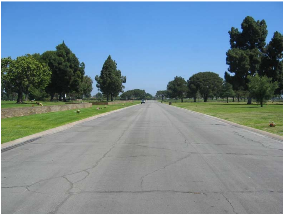
Figure 9. View along the Project ROW on Guardian Drive at Forest Lawn. View toward north. June 25, 2015.
